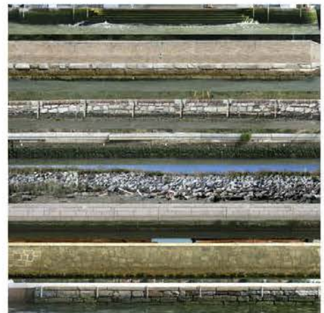
[7] FROM THE TOP, THE WATERFRONTS OF: ZATTEREGESUATI, THE NAPOLEONIC GARDENS, SANT'ERASMO SOUTH, SAN GIULIANO EAST, SANT'ERASMO NORTH, SAN GIULIANO WEST, MURANO-SACCA SERENELLA, LIDO-ALBERONI.
