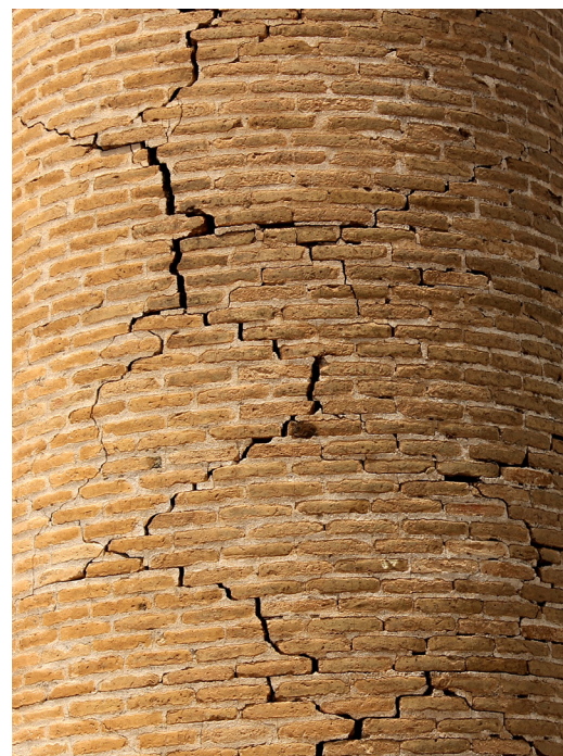
Figure 8: Detail of the textured model showing the cracks of the chimney (source: prepared by the authors)
