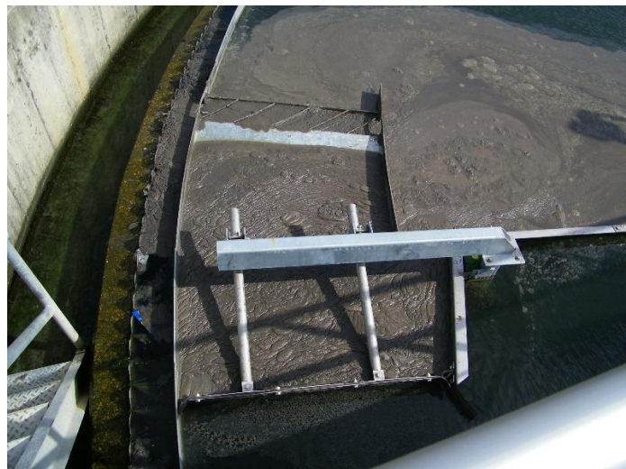
Figure 21: Primary clarifier picture
