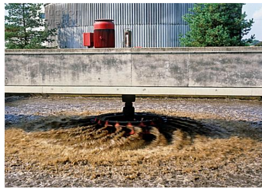
Figure 22: Aeration tank picture
