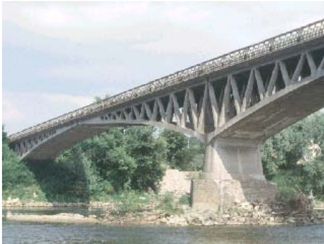
Figure 2.4 Boutiron Bridge. The only of the three similar built that survived World War II.
