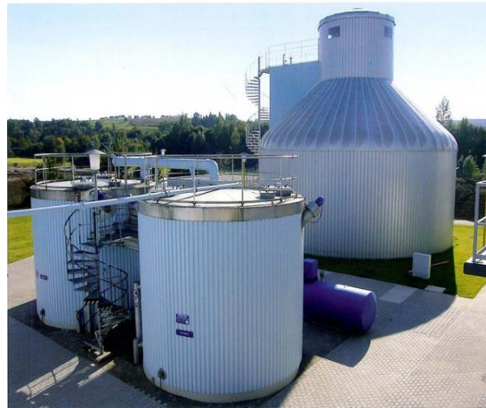
Image 9. Stripping treatment plant
