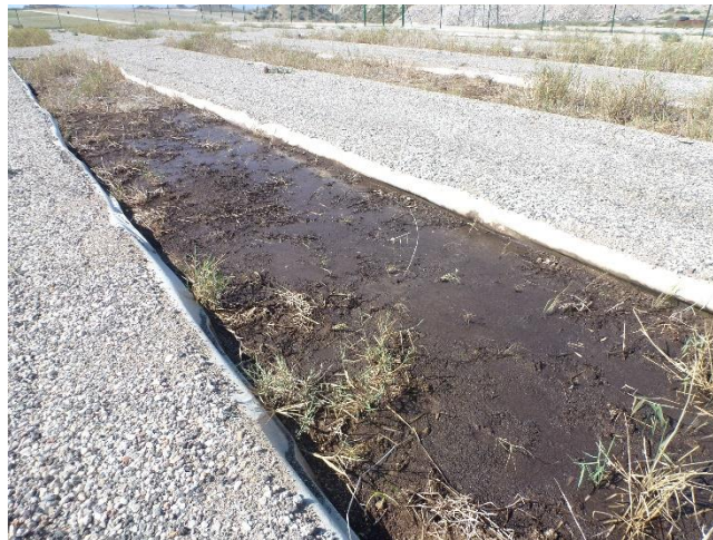
Photo 2. Clogging of the constructed wetland
