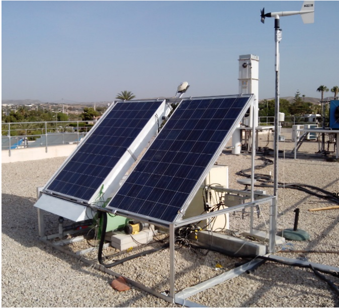
Figure 2: Prototype of Photovoltaic Evaporative Chimney.
