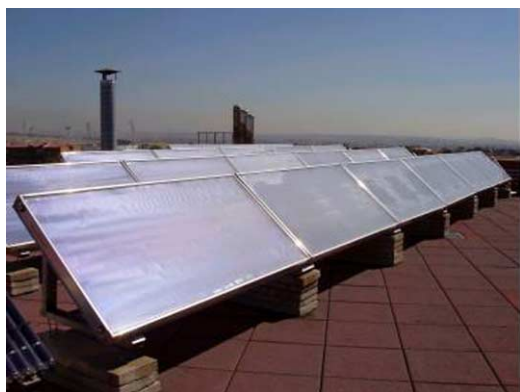
Fig. 2. View of the flat-plate solar collector array installed on the roof of UC3M Leganés Campus.
