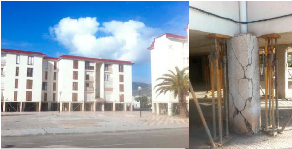
Figure 9. Overview of the San Fernando neighborhood after the 11 May 2011 earthquake [6]. Widespread damage can be observed in columns on the ground floor.
