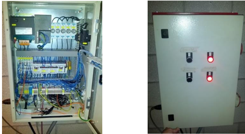
Fig. 57. - a,b Communication Cabinet
