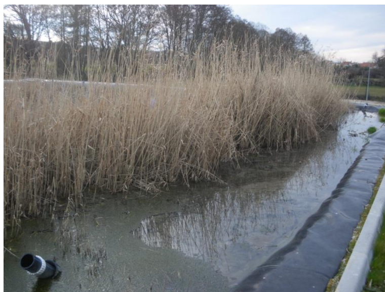
Picture 14. Bed colonized with Phragmites australis , in the subsurface horizontal flow of a constructed wetland (HSSF CW) located at Vila Fernando .
