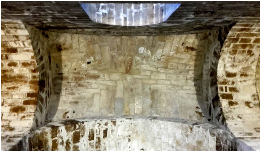
Fig. 10 Groin vault with linear—not “L” shaped—voussoirs solution in edges. Church of San Cataldo (Palermo, c. 1154). Photo: authors, 2016
