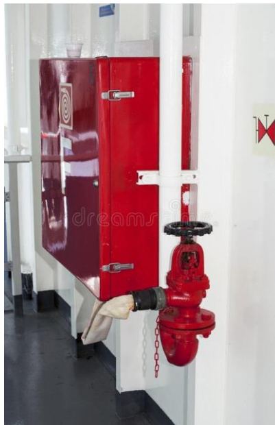
Figura 43. Hidrante y puesto de incendio. Fuente: https://www.dreamstime.com/water-hose-hydrant-box-fire-protection-system-ship-fire-protection-system-ship-service-station-factory-industry-image205223306
