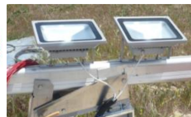
Figura 10: Foco LED (carga)
