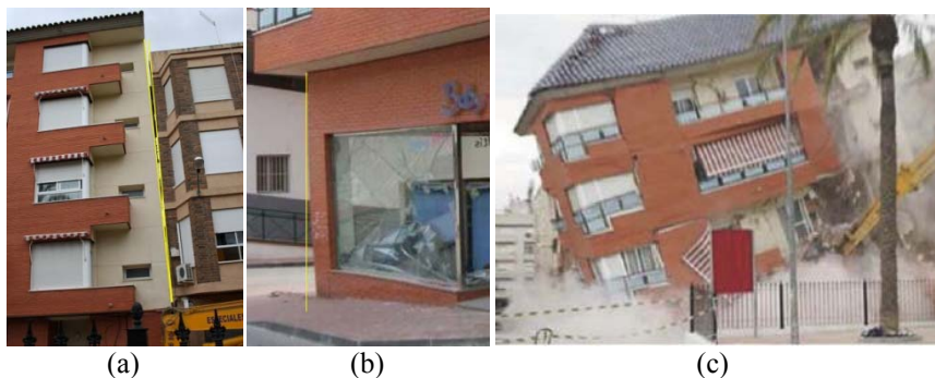
Figure 8. Building in danger of collapse. Evidence of crashes in (a) joint between buildings and (b) corner pillar. (c) Collapse.
