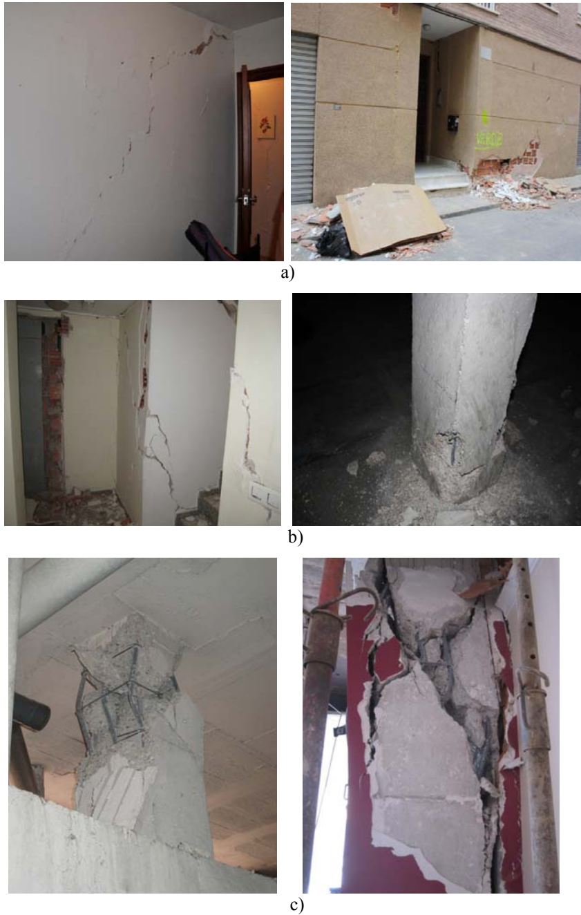
Figure 4. Damages in structural and non-structural elements of buildings after the Lorca earthquake, 2011 typically labelled as a) green label, b) yellow label or c) red label. Source: Authors.
