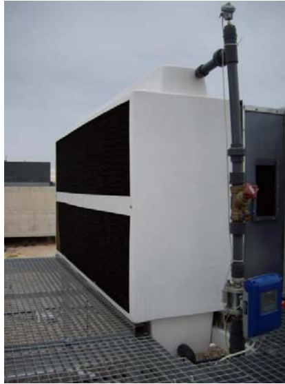
Figure 1: Experimental cooling pad setup.
