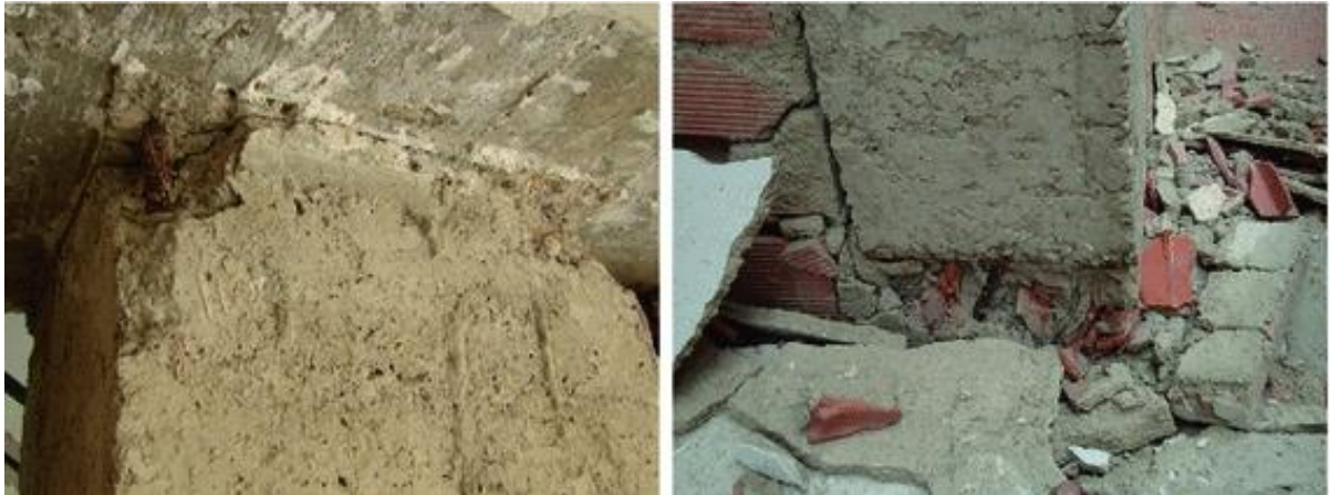
Figure 14. Examples of failure at the construction joint of a beam-column connections.
