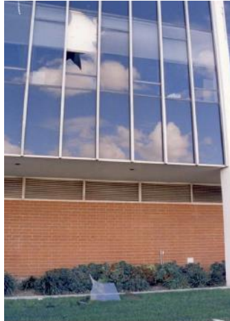
Figure 41 Shards of window pane, 1994 Northridge Earthquake (Robert Reitherman, 2009)
