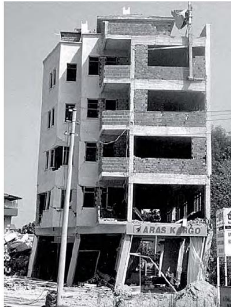
Figure 16 example soft-storey ground floors [3]
