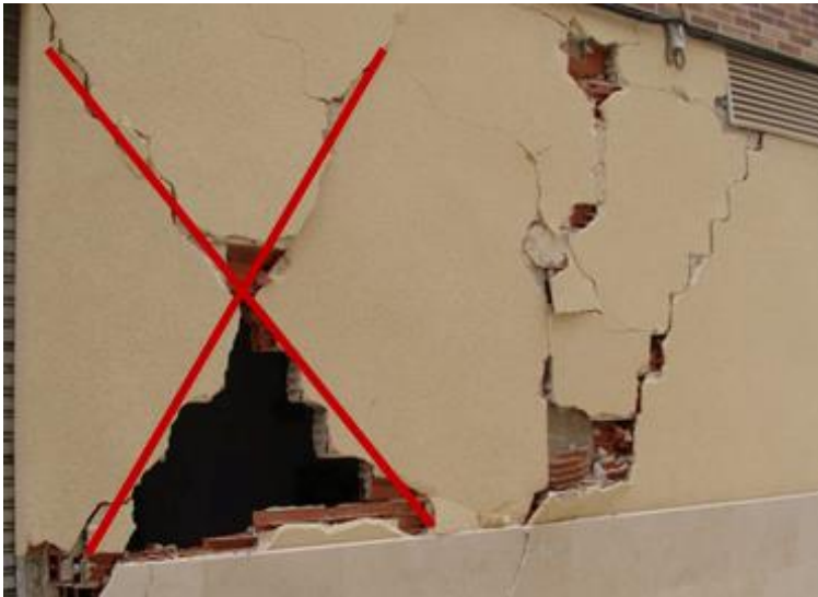
Figure 142 Typical break in a wall due to earthquake
