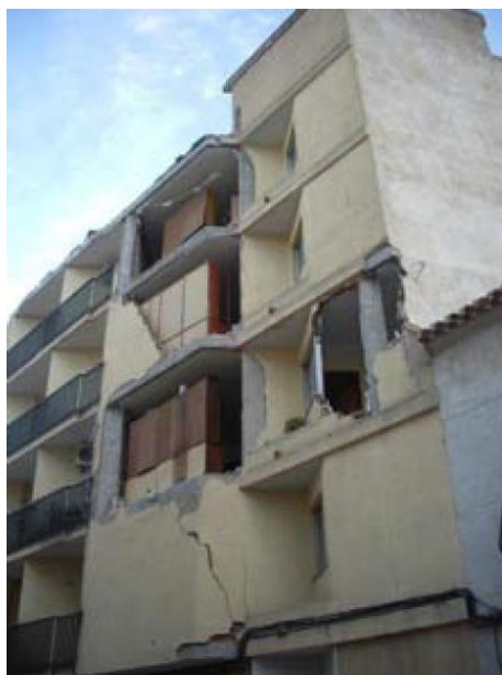
Figure 30 Building damaged by pounding in Lorca earthquake (Informe del Sismo de Lorca del 11 de Mayo de 2011)
