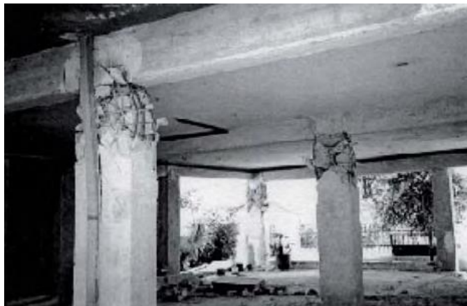
Figure 17 damage at ends of pillars of soft-storey ground [4]
