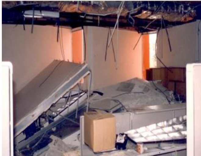
Figure 39 Failure of office partitions, ceilings, and light fixtures in the 1994 Northridge Earthquake (FEMA 74, 1994).
