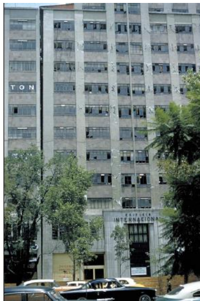
Figure 42 Drift-caused damage to windows in the International Building in Mexico City in the M 8.1, September 19, 1985 Mexico Earthquake (Robert Reitherman, 2009)
