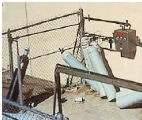
Figure 43 Overturned medical gas cylinders, 1971 San Fernando Earthquake (Scientific Service, Inc.)
