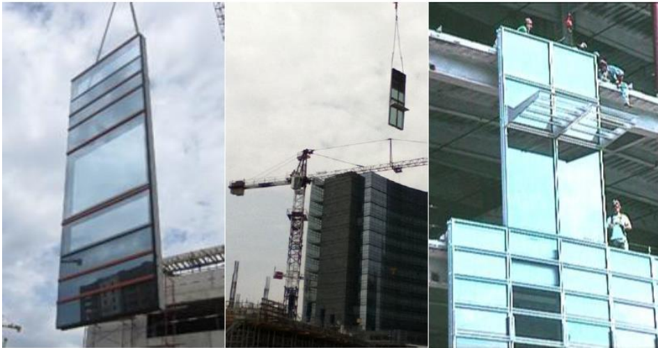
Figure 110 Several moments during the installation phase of a unitized curtain walling system (Umberto GALLI, 2011)
