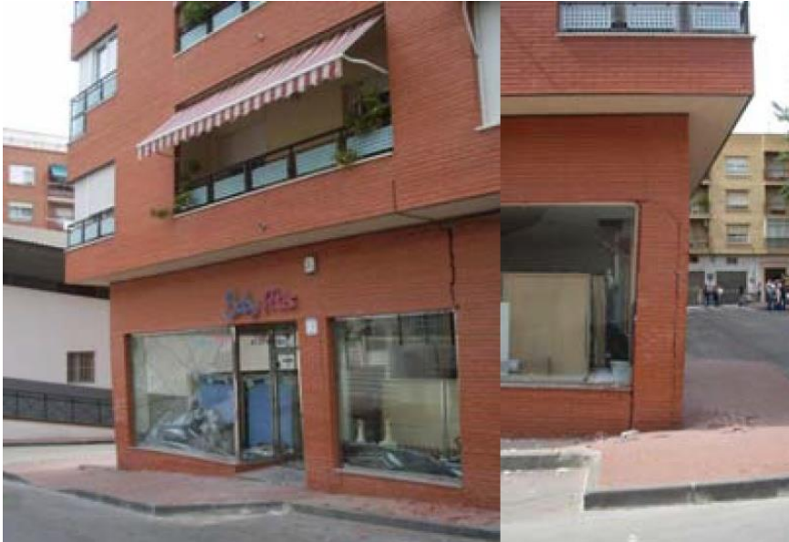
Figure 25 torsion by the stiffening effect of the dividing walls in Lorca earthquake 2011 (Informe del Sismo de Lorca del 11 de Mayo de 2011)
