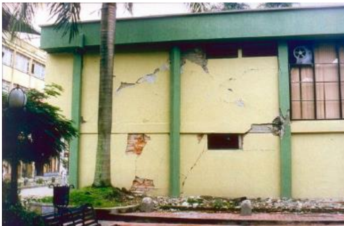
Figure 61 Major damage to the unreinforced masonry infill walls and moderate damage to the columns of an R/C municipal building (Quindia, Colombia 1999 Earthquake, EERI).
