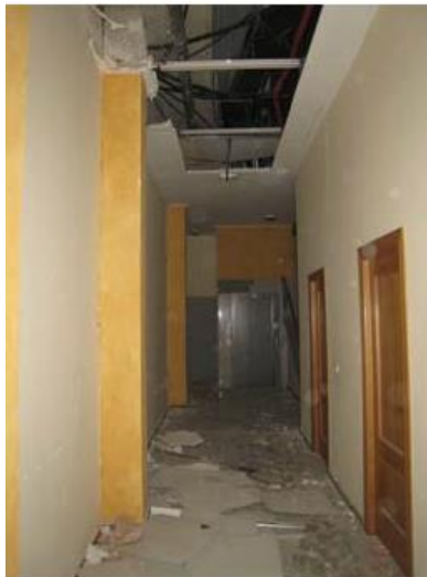
Figure 38 Failure of suspended ceilings and light fixtures in Lorca earthquake 2011 (Tomas Espín, 2011)
