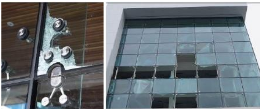
Figure 116 Examples of damage to spider glazing systems (Andrew Baird et al, 2011)
