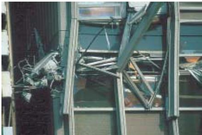
Figure 22 crushed upper floor of the office building (Kobe, Japan 1995).
