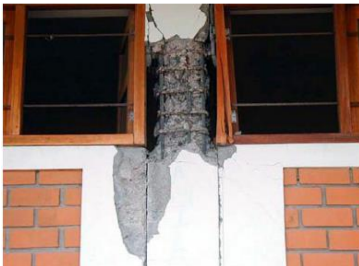
Figure 62 Short column effect due to partial tight fit infill walls in an R/C building (Arequipa, Peru, June 2001 Earthquake, EERI).
