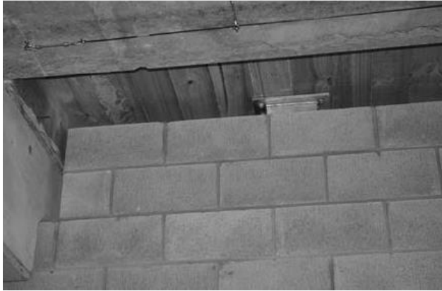
Figure 65 A reinforced masonry infill wall separated from surrounding structure.
