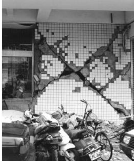
Figure 58 Typical infill wall diagonal crack pattern. 1999 Chi-chi, Taiwan earthquake.
