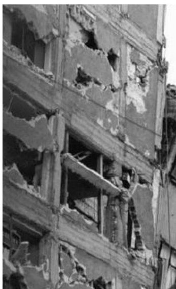
Figure 57 Damage to the tops of several columns due to infill wall compressive strut action. Mexico City, 1985 Mexico earthquake.
