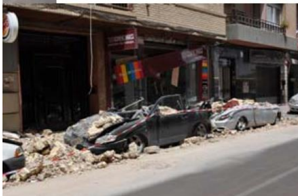
Figure 36 Failure in the cornice of a building in Lorca Earthquake 2011 (Tomas Espín, 2011)
