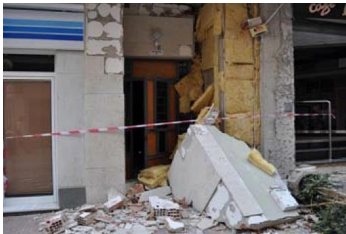
Figure 34 Failure Cladding of a building in Lorca Earthquake 2011 (Tomas Espín, 2011)
