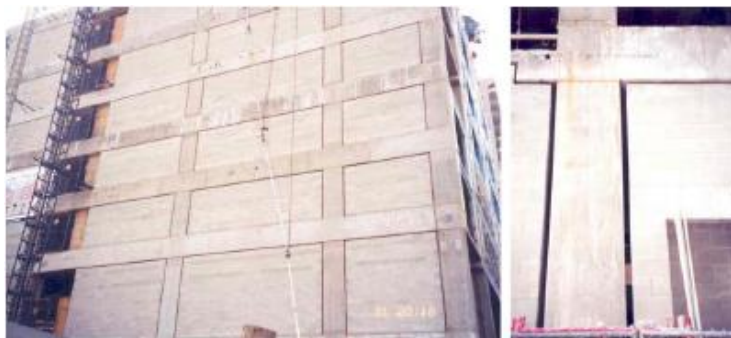
Figure 63 Isolated infill walls from R/C frame with gaps in a recent construction.
