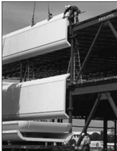
Figure 93 Erection of precast concrete panels with push-pull connections (Chris Arnold et al, 2009)
